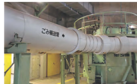
廃棄物空気輸送管 Pneumatic trash-carrying ducts
