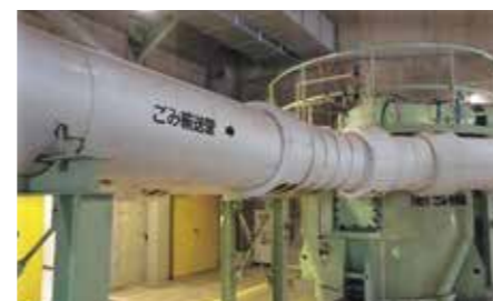
廃棄物空気輸送管 Pneumatic trash-carrying ducts
