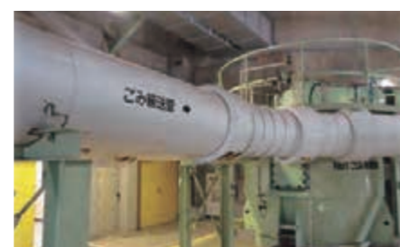
廃棄物空気輸送管 Pneumatic trash-carrying ducts
